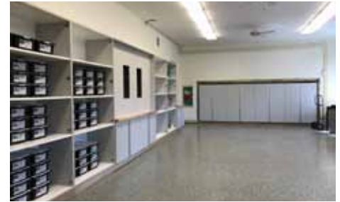
The creation of the Innovation Lab began with the installation of hybrid polymer floors and customized shelves and storage cabinets.
